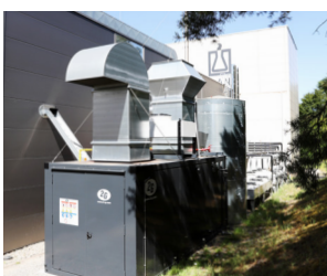
Combined heat and power unit
